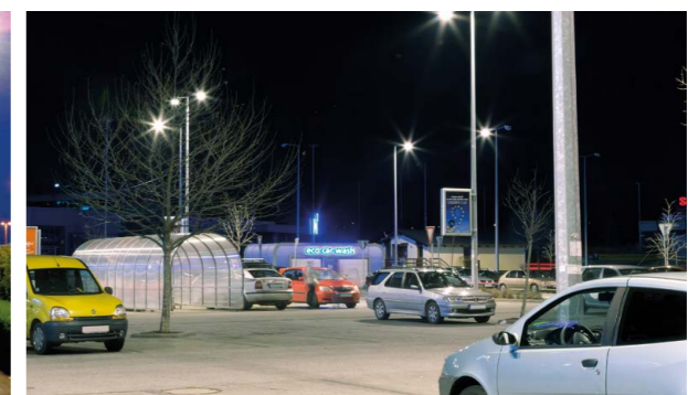
In larger car parks, it is better to mount multiple luminaires on each pole and at higher mounting heights. This reduces the infrastructure required.
