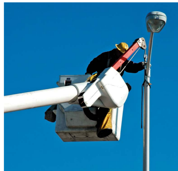
Maintaining and changing light sources in streetlighting applications is a complex, costly and often inconvenient task.
