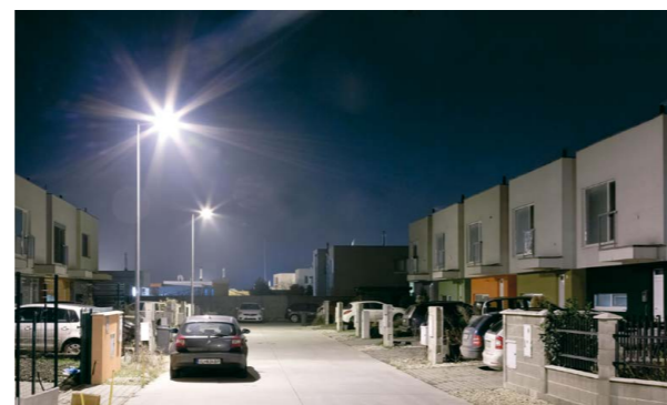
The white light is more focused where needed and appears brighter and more natural, promoting safety. The new installation is also much more efficient.
