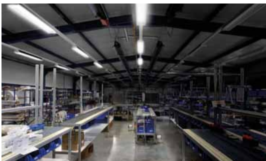
At times with limited activity in the space it is possible to switch on only the luminaires needed in the necessary location by selecting the suitable lighting scene.
