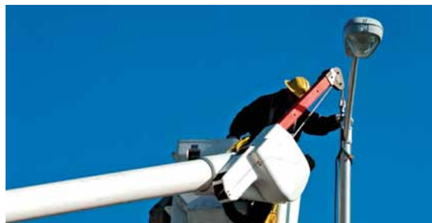
The removal of old luminaires, light sources, wiring and materials requires safety and professionalism. If you choose, we can also arrange the recycling of all waste materials.
