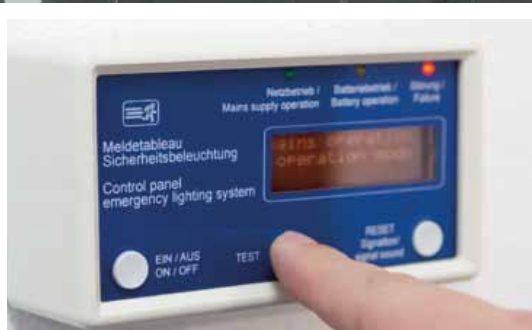
Larger lighting installations need to incorporate a central monitoring system from where the lighting functionality can be remotely tested.
