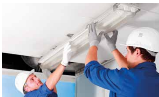
For luminaires to work without any trouble it is important to connect them properly under the supervision of professionals.
