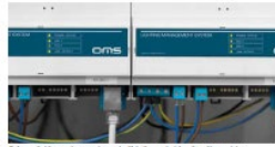
Before a lighting system can come to life, the control functionality must be programmed.
